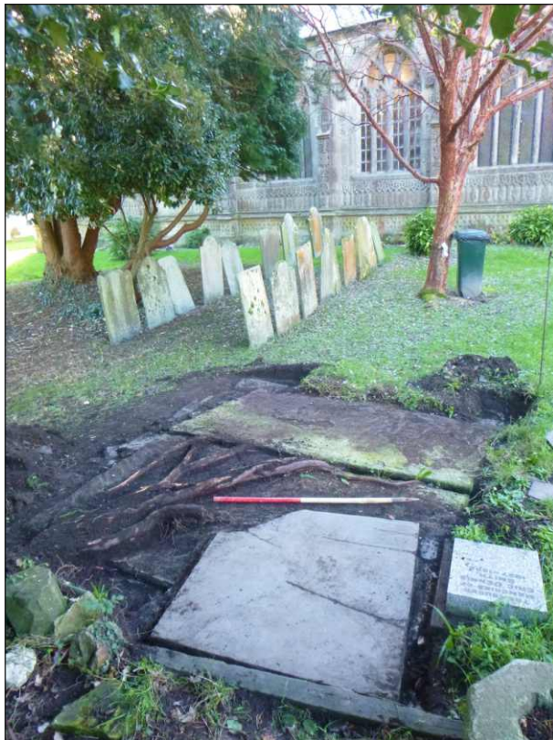
Plate 2: View of intrusive tree roots, concrete capping and later slate slab forming the repair dating to after 2004, looking southwest (1m scale)
