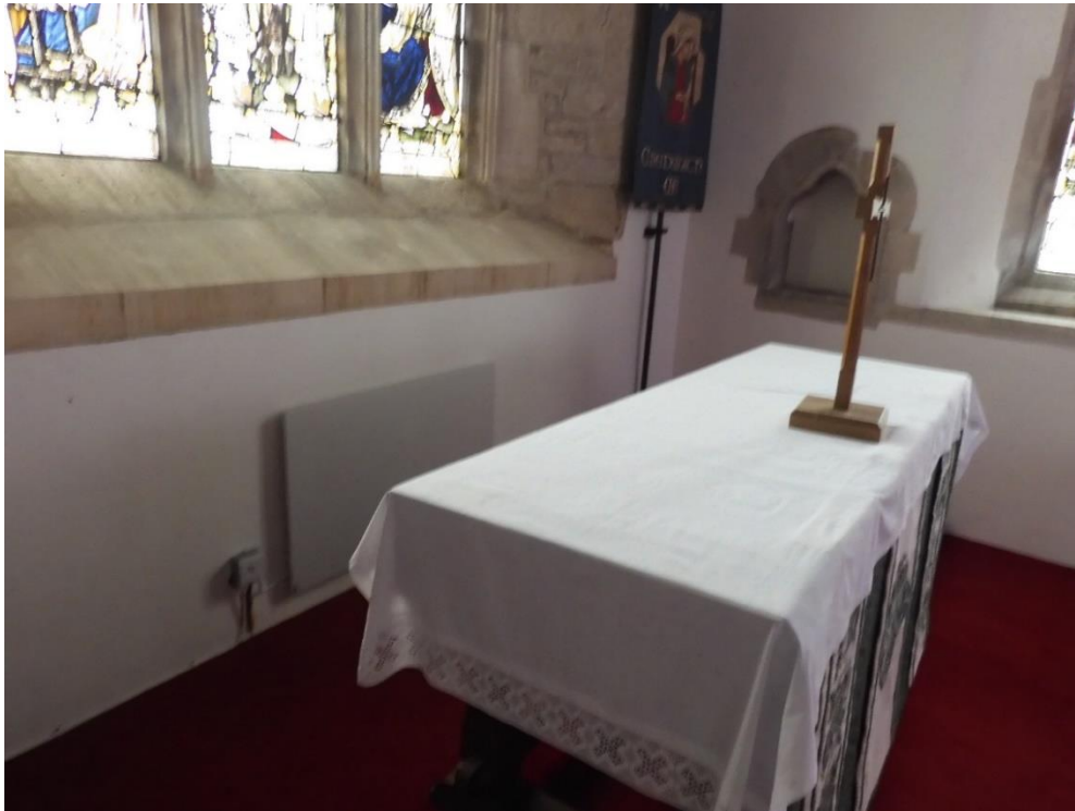
Electric panel heater installed behind an altar
