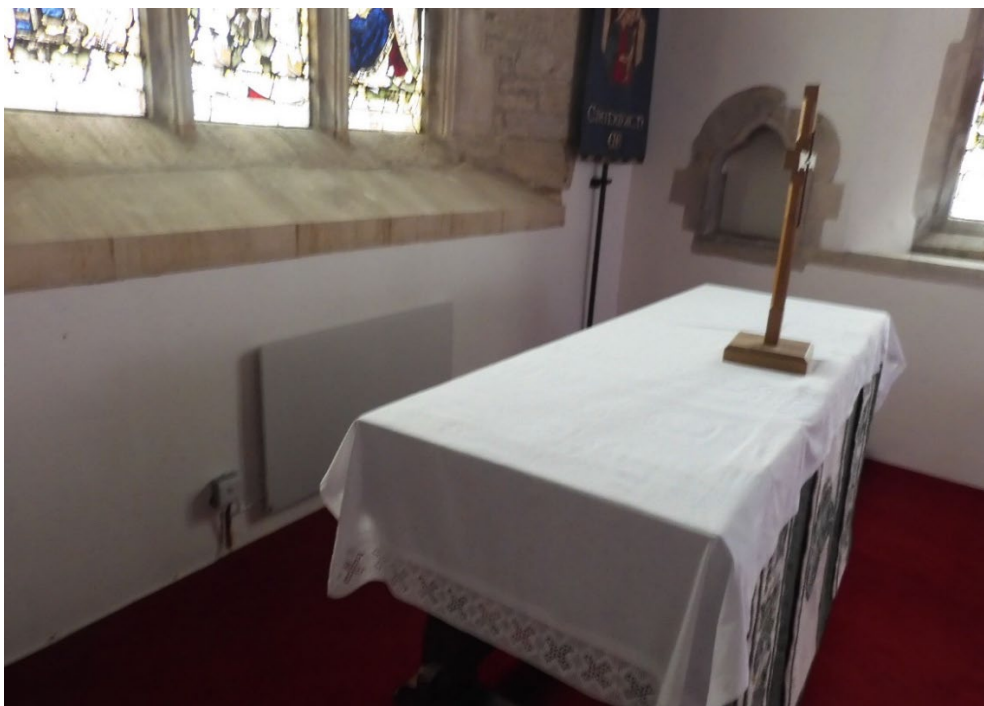
Electric panel heater installed behind an altar
