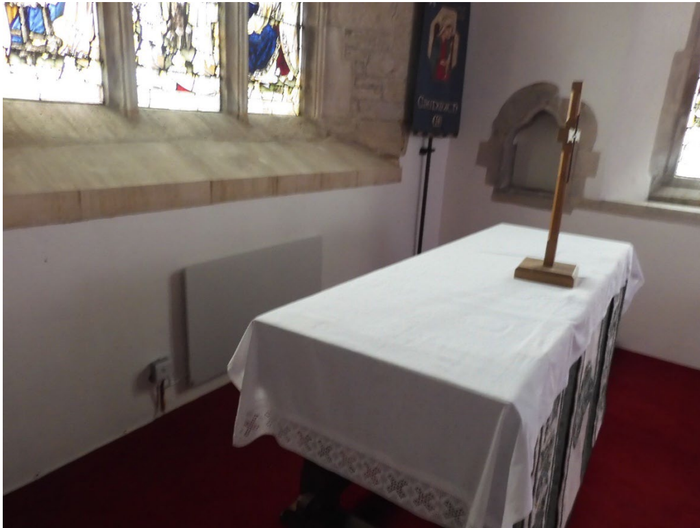
Electric panel heater installed behind an altar
