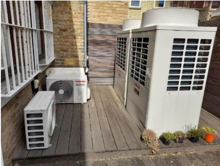
Examples of external units for ASHP comprising of three smaller 3kW units (output 10kW each) and two larger 10kW units (output 37.5kW each).
