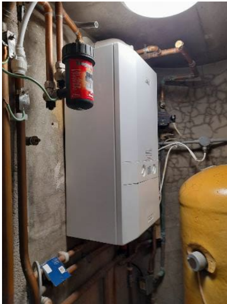
Sports Hall office area boiler.
