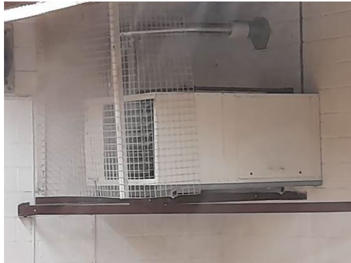
Sports hall gas space heater.
