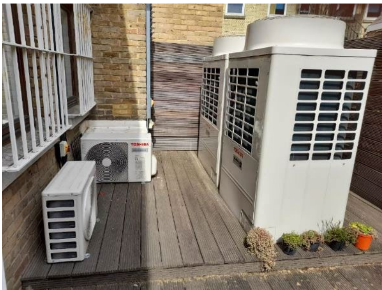
Examples of external units for ASHP comprising of three smaller 3kW units (of 10kW output each) and two larger 10kW units (of 37.5kW output each).
