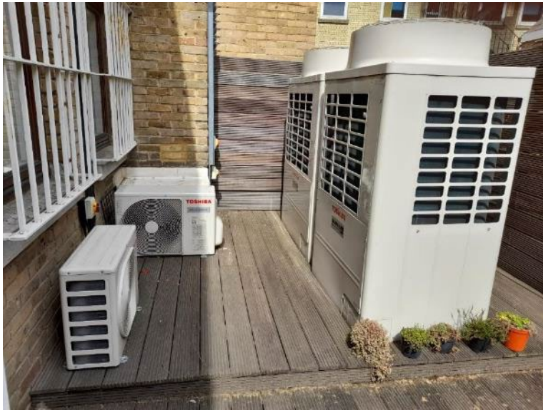
Examples of external units for ASHP comprising of three smaller 3kW units and two larger 10kW units which supply 37.5kW of heat each.
