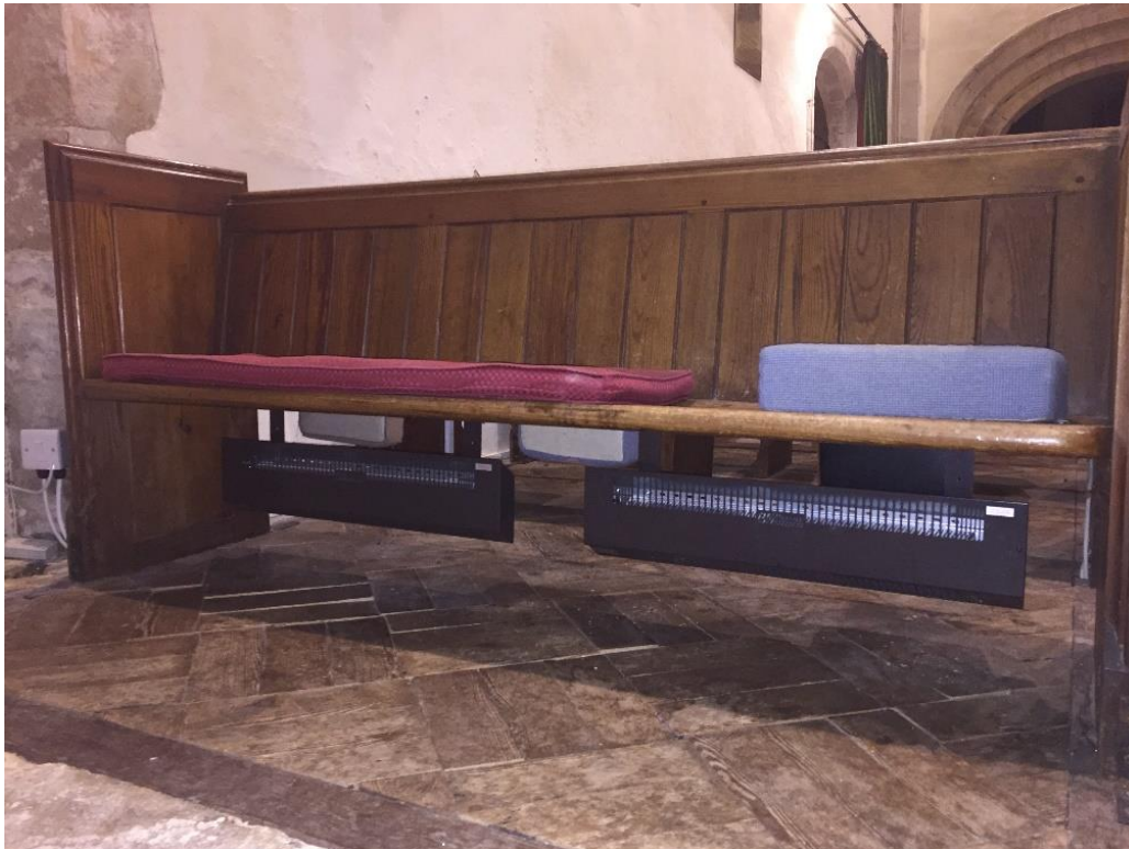
Brown BN Thermic 650W under pew heaters fixed to underside of pew seats for pews which have no solid backs.
