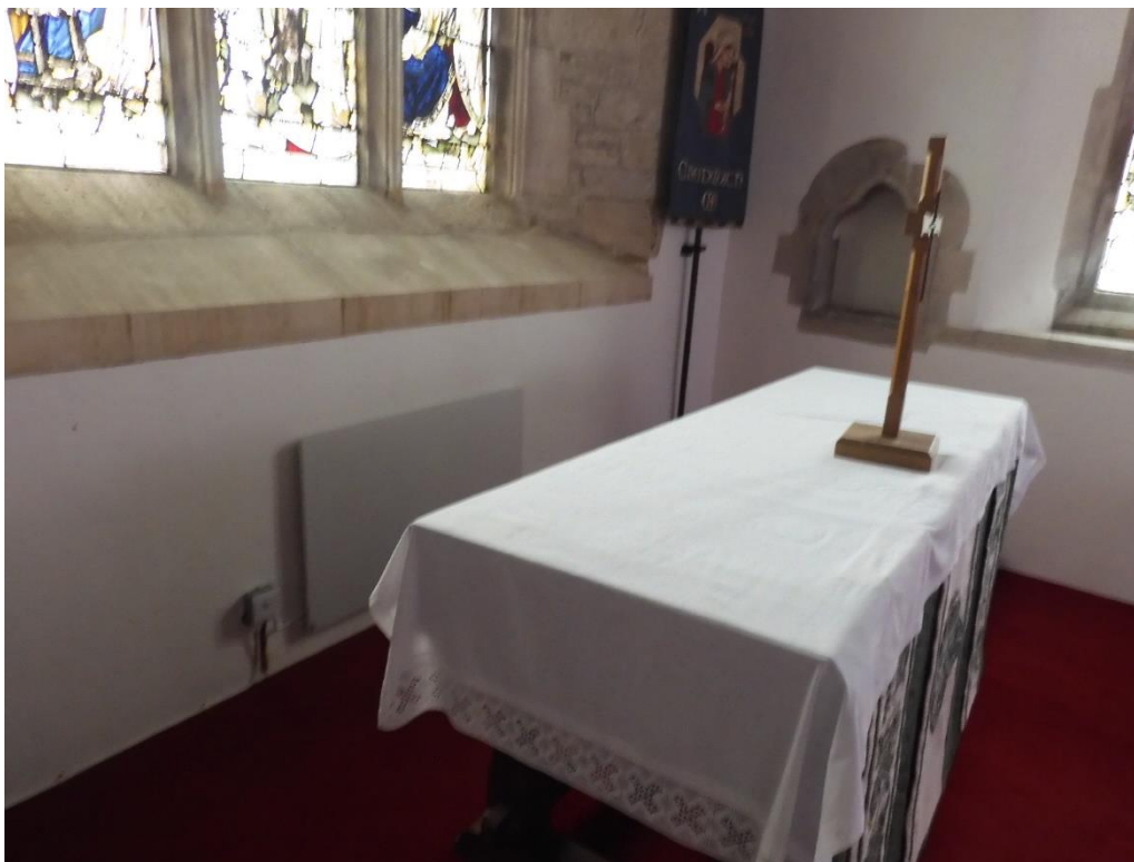
Electric panel heater installed behind an altar
