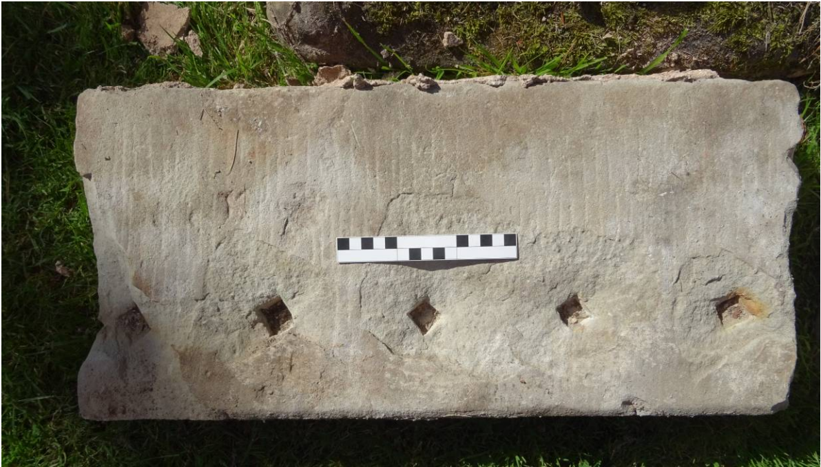
Plate 24. A broken section of a kerb (plinth) with railing footings
