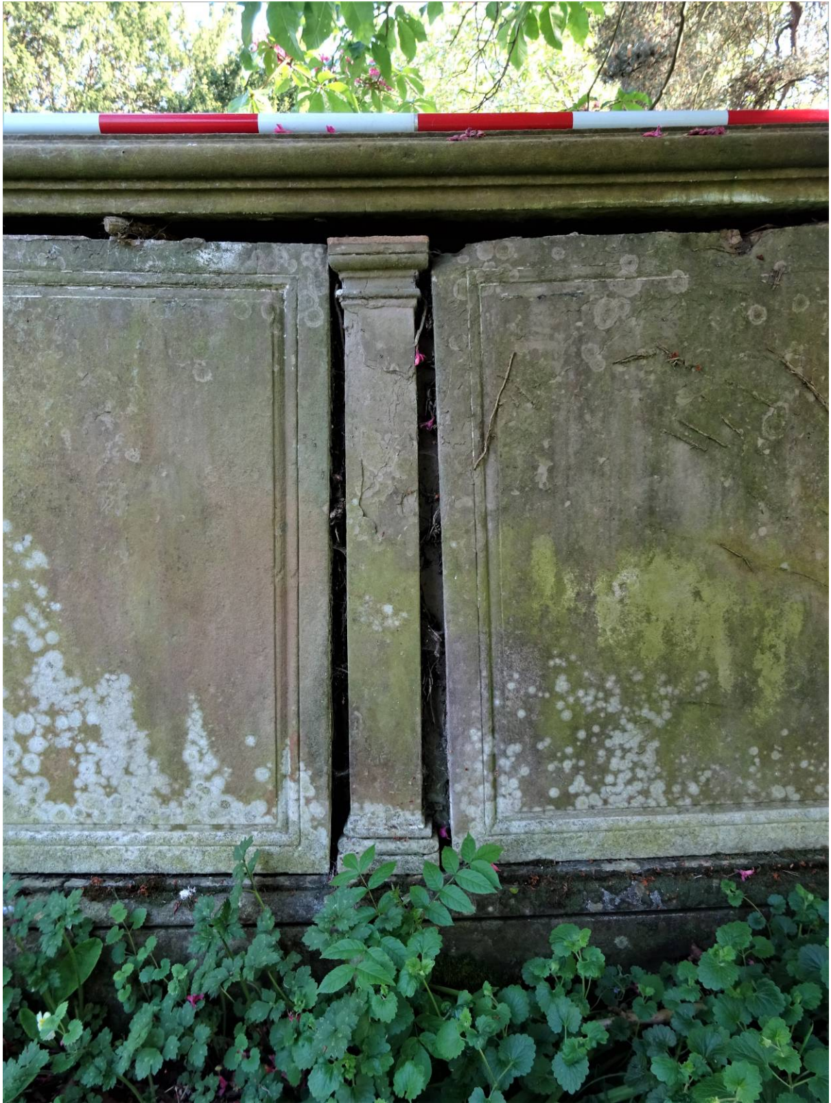
Plate 6. View of the central column on the northern side of the tomb
