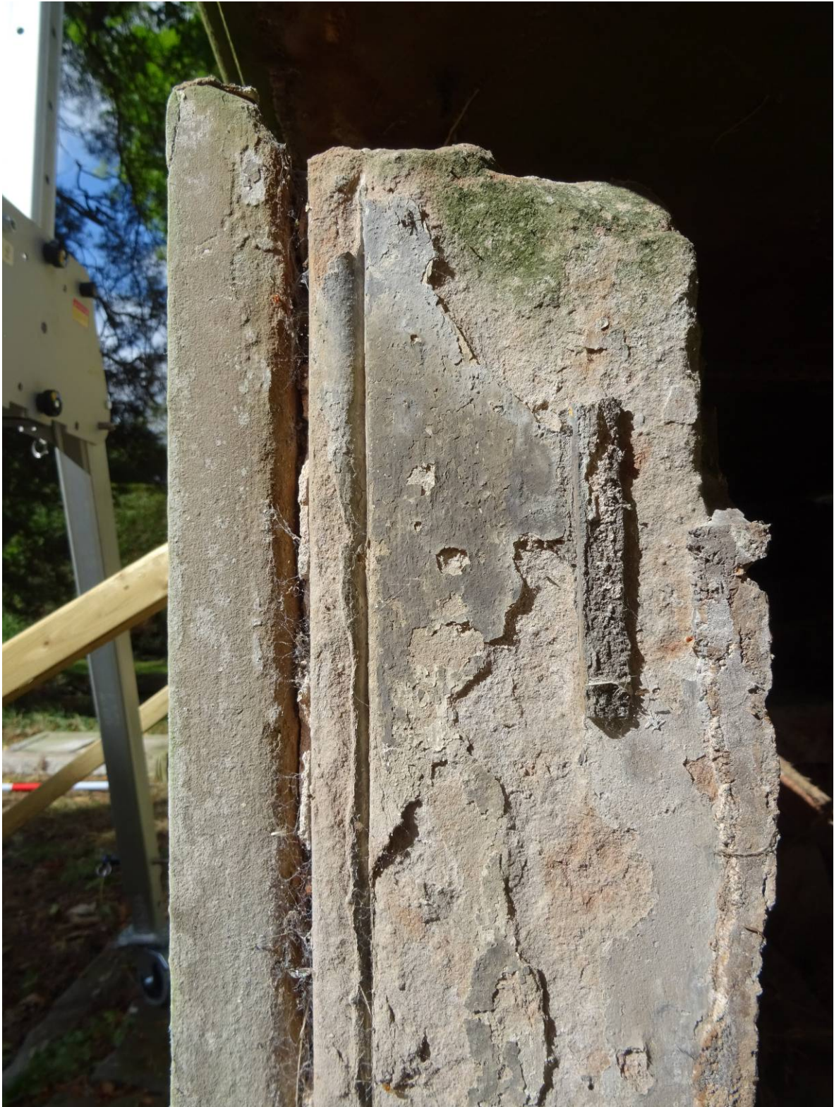
Plate 13. Stone column with the trace of an iron fitting and a later cement regime
