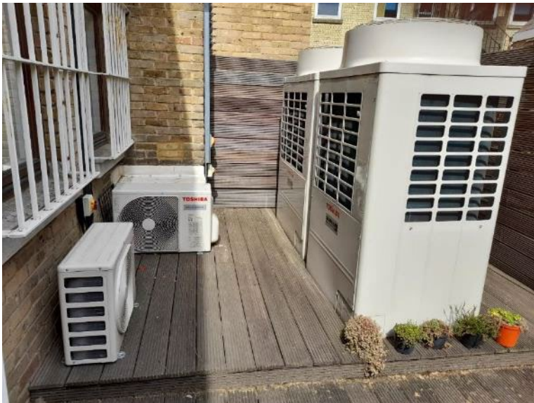
Examples of external units for ASHP comprising of three smaller 3kW units with 10kW output each and two larger 10kW units with 37.5kW output each.
