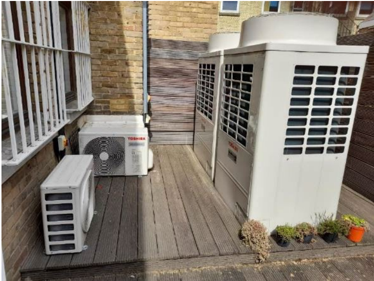
Examples of external units for ASHP comprising of three smaller 3kW units delivering 10kW heat each and two larger 10kW units delivering 37.5kW of heat each.
