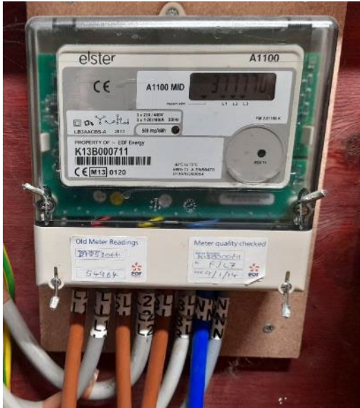
Above, church electricity
