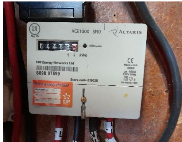
Above, office electricity
