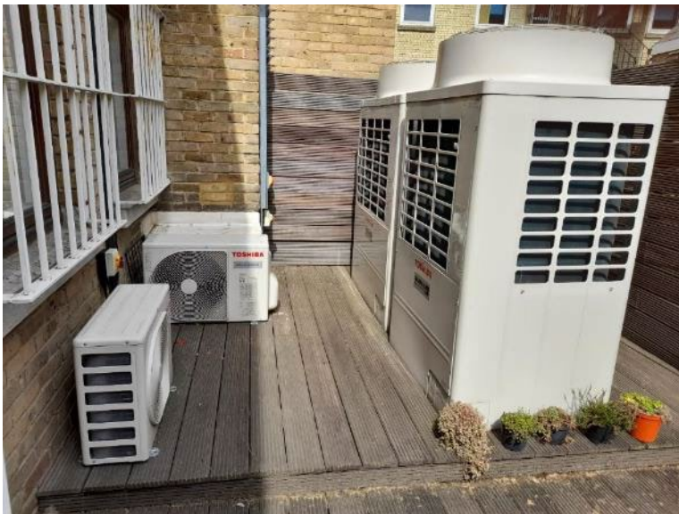
Examples of external units for ASHP comprising of three smaller 3kW units (10kW output each) and two larger 10kW units (37.5kW output each). Together they supply a building of 660m 2 .
