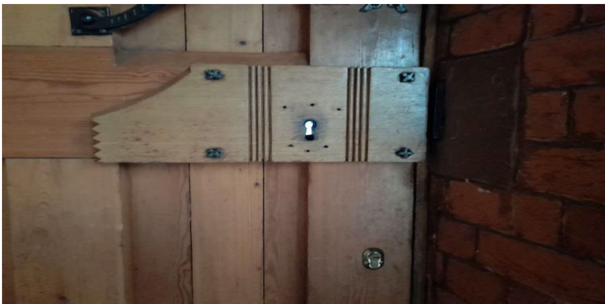
The choir vestry door keyhole could be addressed using a small cover affixed by blu tack.
