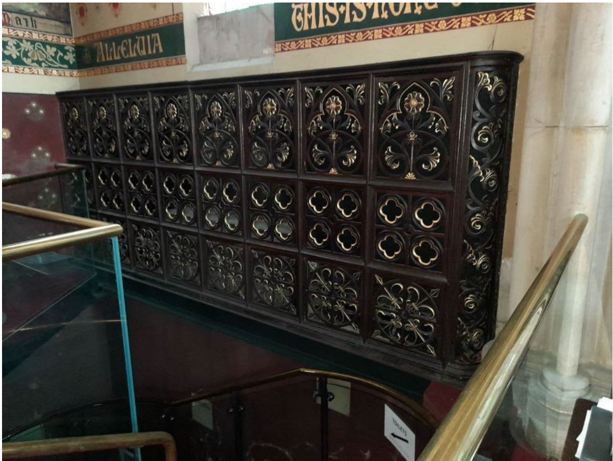
Two further fan assisted radiators are hidden inside these metal screens at the rear.
