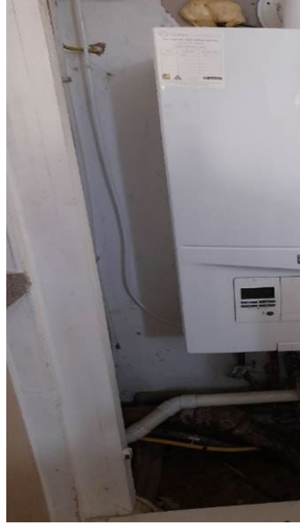
Crypt boiler, 28kW
