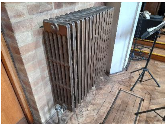
Radiator in nave
