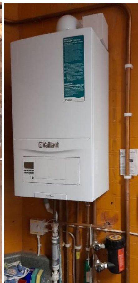
Office and undercroft boiler
