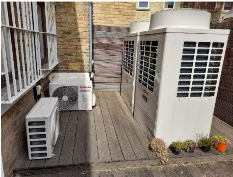
Examples of external units for AASHP comprising of three smaller 3kW units (output 10kW each) and two larger 10kW units (output 37.5kW each).
