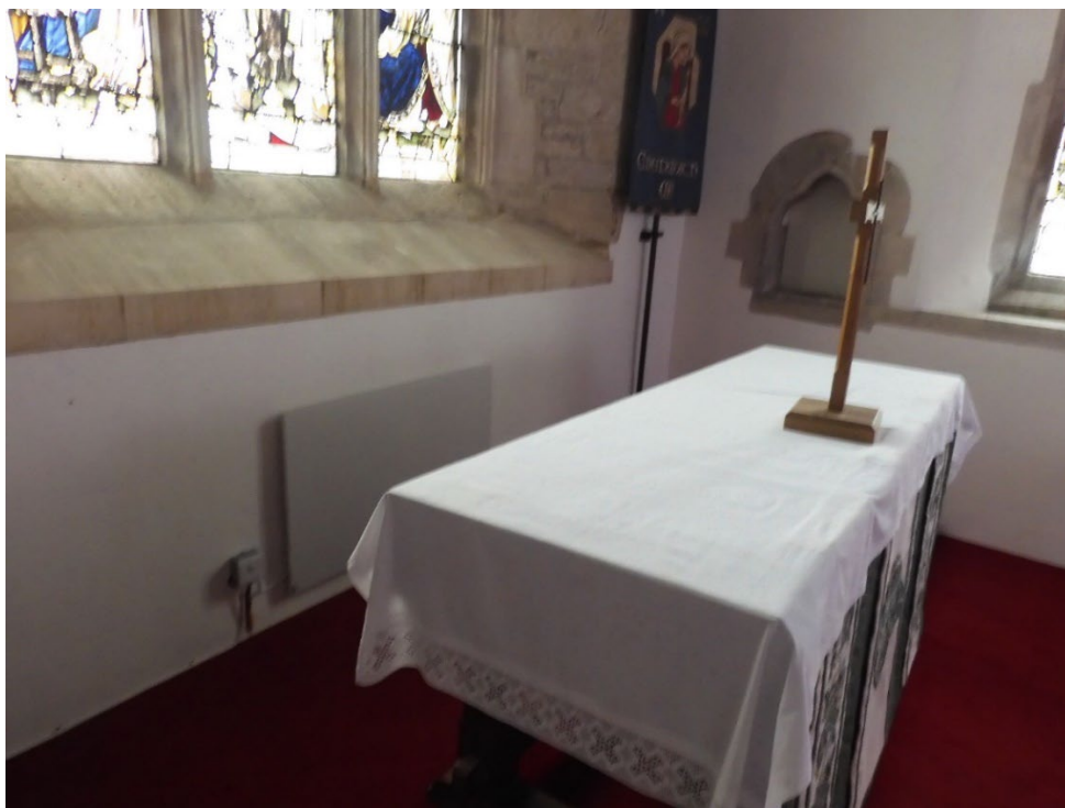
Example of an electric panel heater installed behind an altar in another church.
