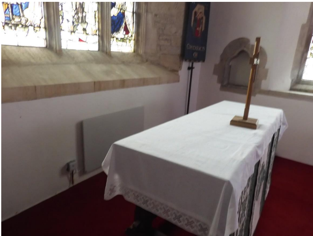
Electric panel heater installed behind an altar
