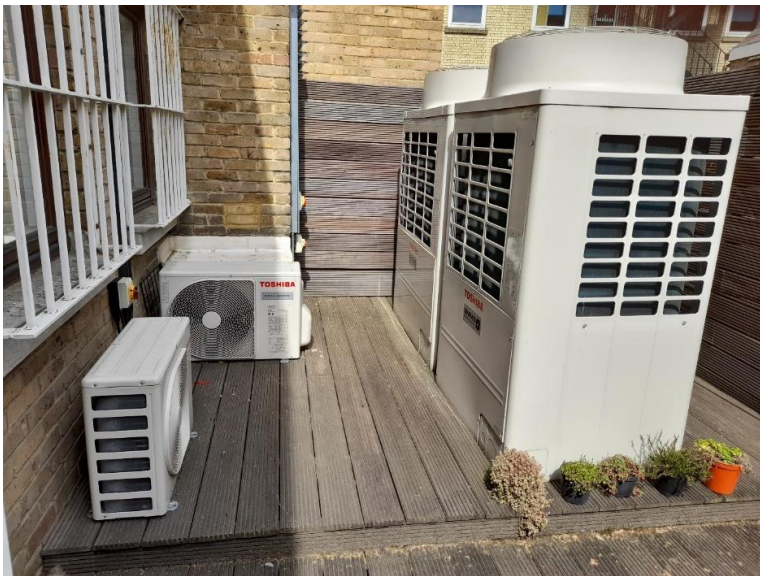
Examples of external units for ASHP comprising of three smaller 3kW units and two larger 10kW units.
