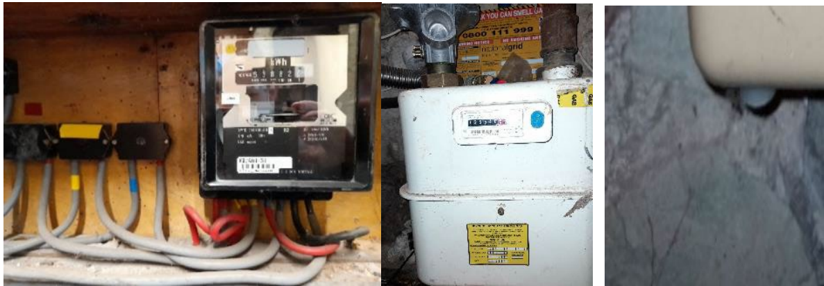
Three phases of power are supplied.
