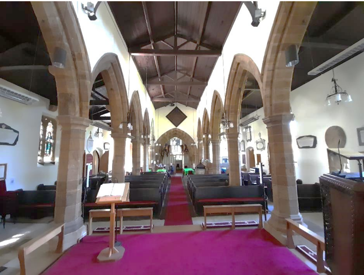
An overview of the church showing the radiant heaters suspended from the arches.
