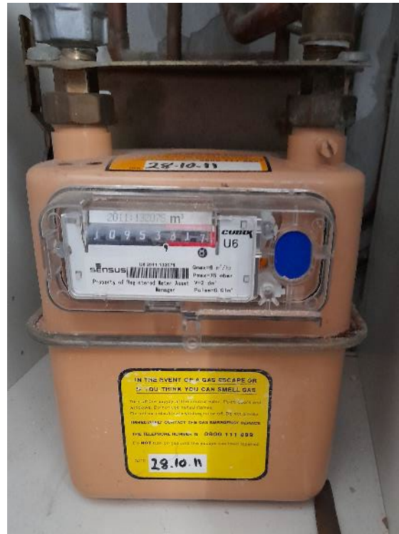
Right, office gas meter
