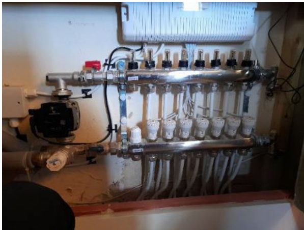
Underfloor heating manifold
