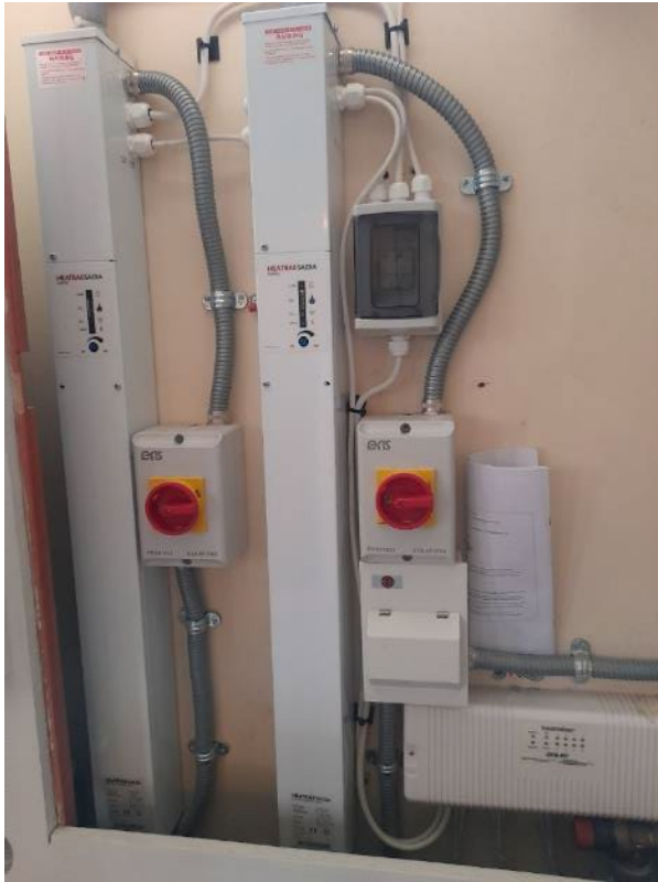
2 x 12kW Heatrae Sadia electric water heaters
