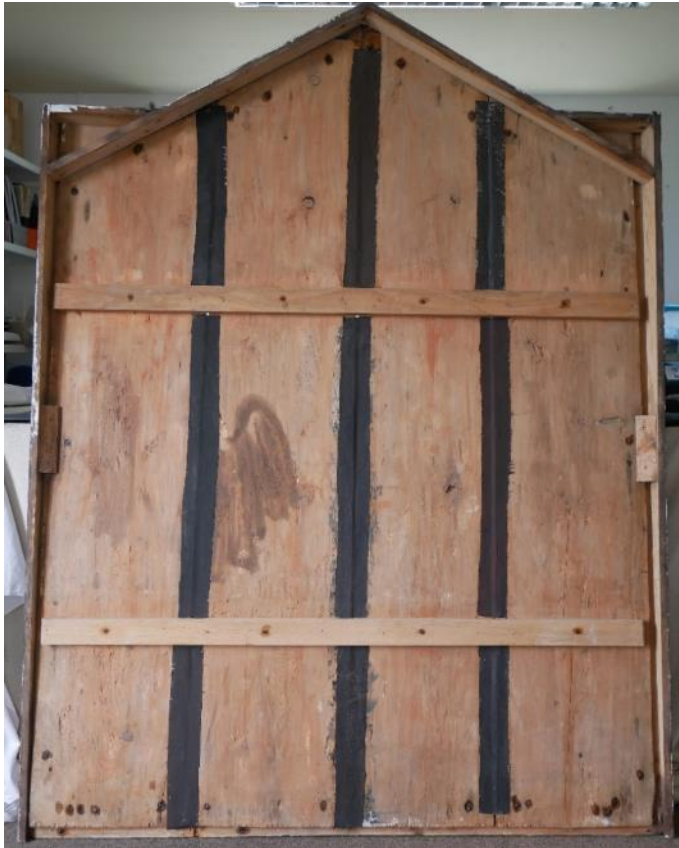
Fig 19 Strips of dark cloth have been glued over the wide gap between the boards to disguise the space. All nail heads and screws were treated with anti corrosive sealant.
