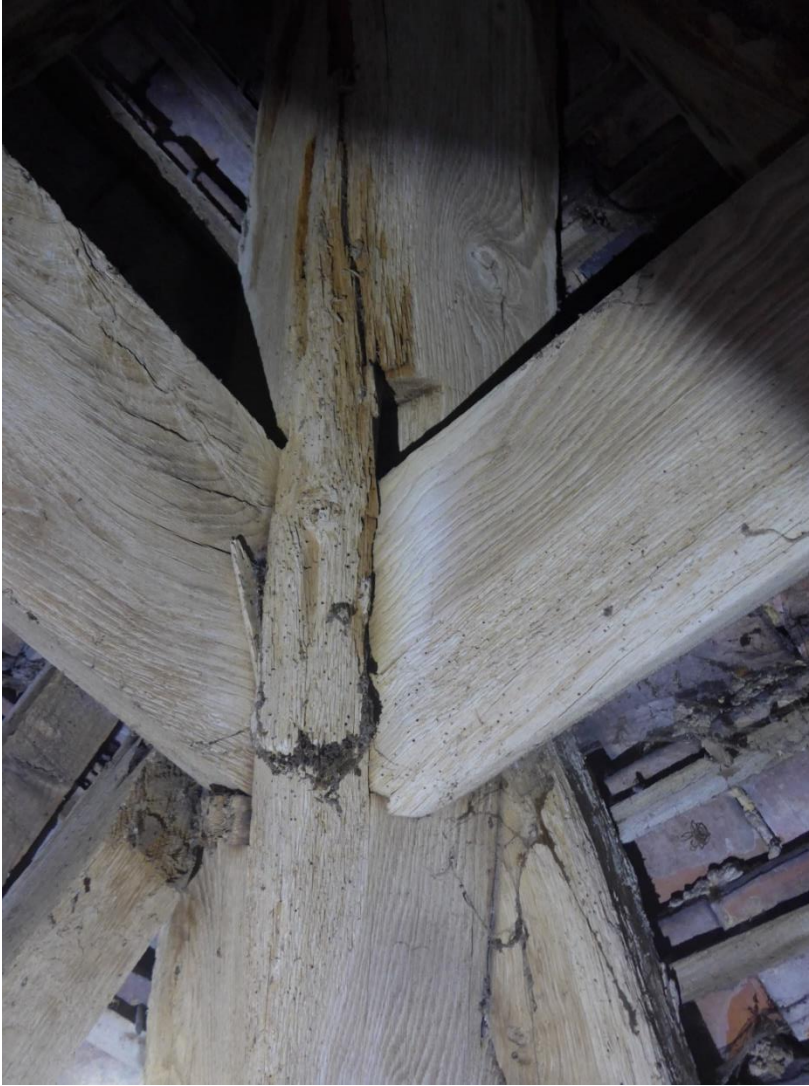
Hip rafter split in NW corner of north chapel. To be plated up to ensure structural integrity.
