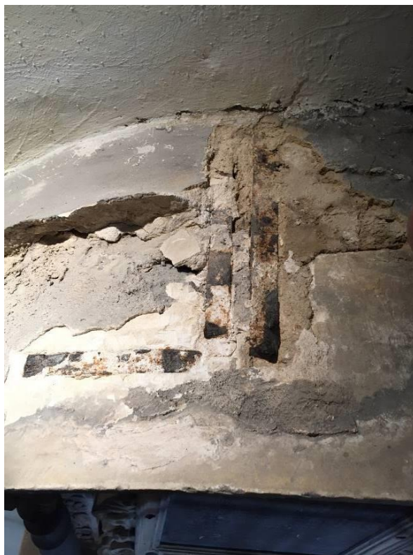
Exposed cramps to west side of pediment
