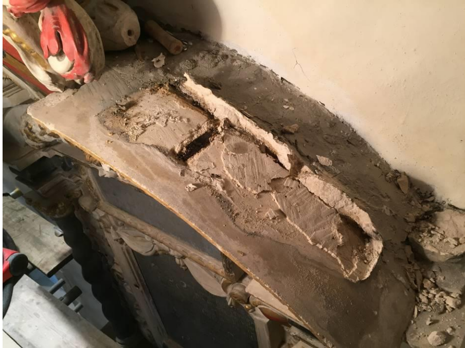
Exposed cramps to east side of pediment
