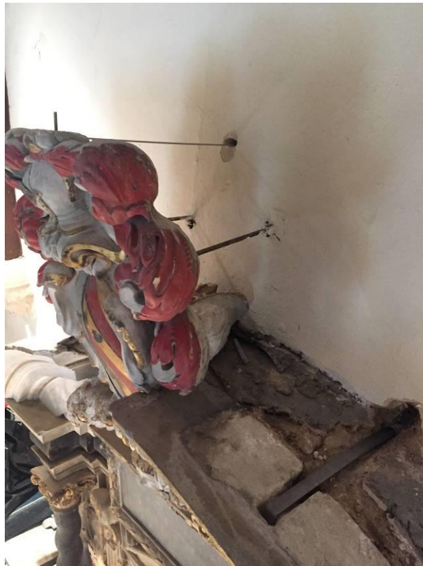
During fitting of east side replacement cramp, shield strap and dowel for crest finial
