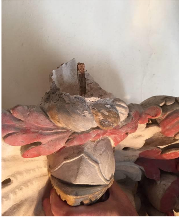
Decayed timber peg for crest finial
