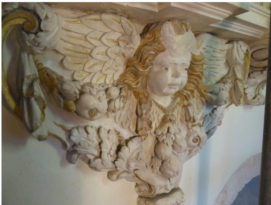
Capping repairs over apron fixings and removal of fixing to cherub head
