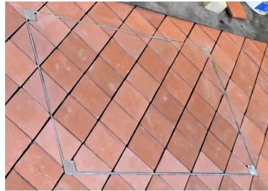
Tiling over a manifold cover:
