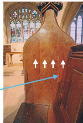
8. View of inside face of the end in Plate 7. Note timber inserts covering hand rail bolt nuts each side of joint between planks
