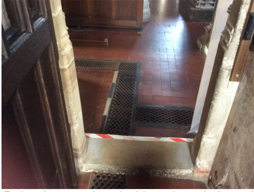
Raised stone threshold to chapel viewed from chapel – trip hazard
