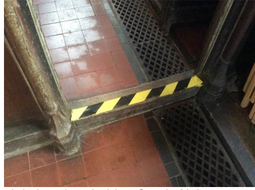
Raised timber threshold to South Aisle screen – trip hazard
