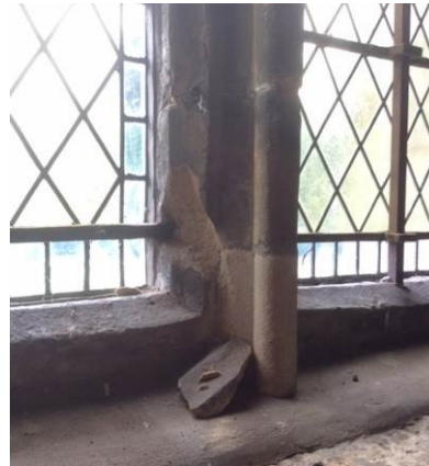
Window Ref No. 6 - corroded embedded ironwork causing cracking and failure of stone
