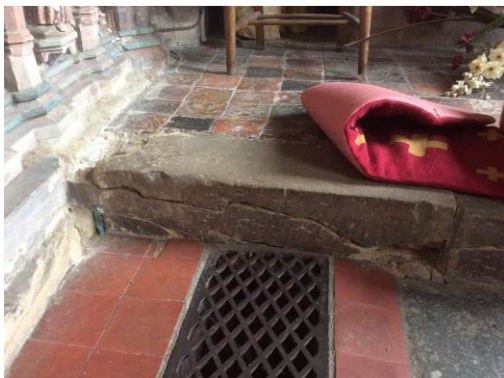
Failing stone to Sanctuary step
