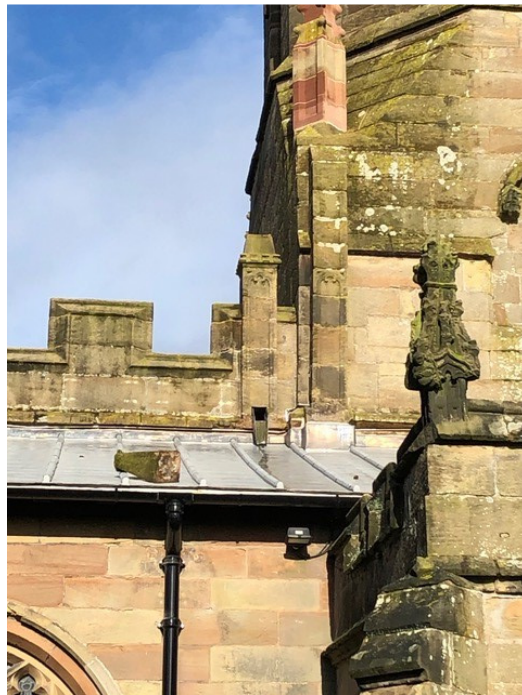
Easterly nave pinnacles – both north and south Both pinnacles are loose, the southerly one recently falling during Storm Dennis.
