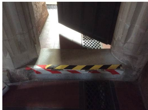
Raised stone threshold to chapel viewed from south transept – trip hazard
