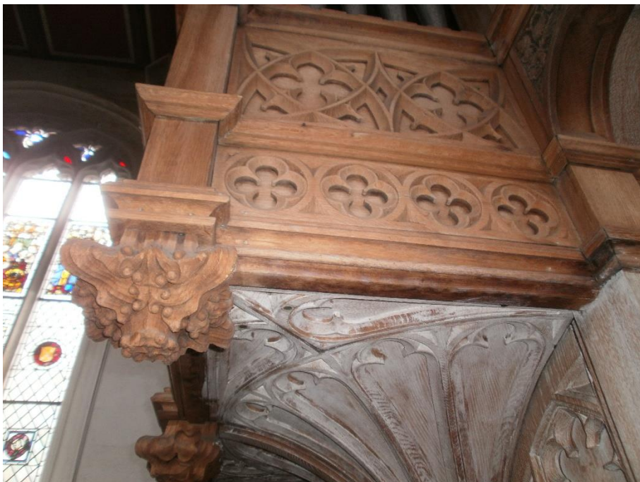
Condition of casework before restoration – part stripped, and part stripped and then heavily limed
