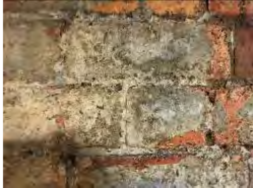
Debris to walls ASC/5 NADIS
