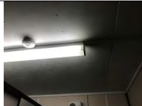
Modern non ACM boards to ceiling
