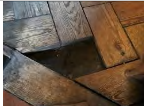
Debris to floor ASC/1 NADIS
