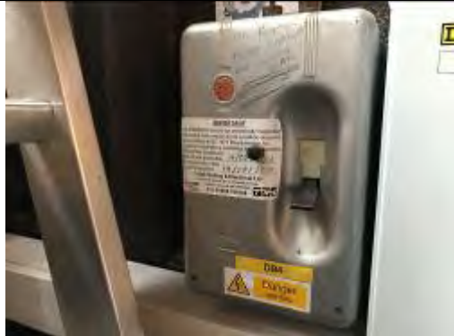
Presumed asbestos flashguards, ropes and seals to older type electrics Chrysotile
