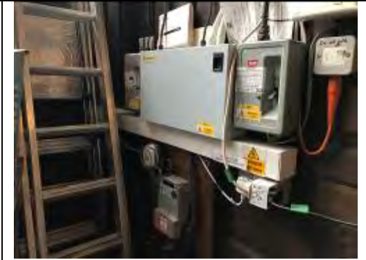
Modern non ACM electrics to left hand side
