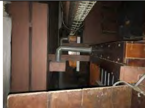
Presumed asbestos insulation board to organ blower box Crocidolite
