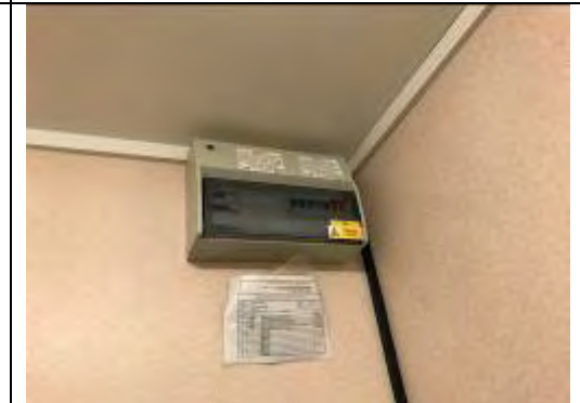
Modern non ACM electrics
