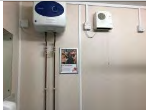
Modern non ACM water heater
