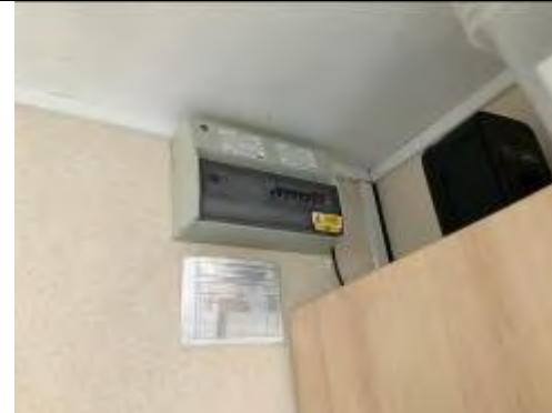
Modern non ACM electrics
