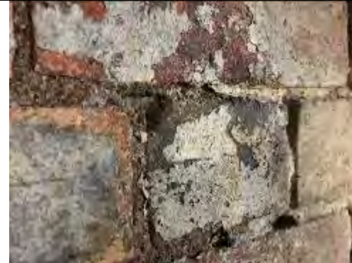
Debris to walls ASC/5 NADIS
