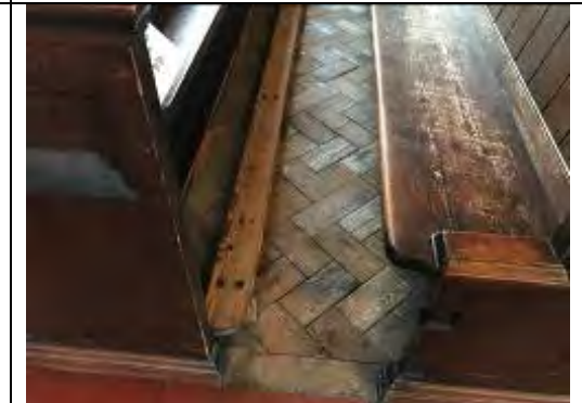
Timber to be removed
