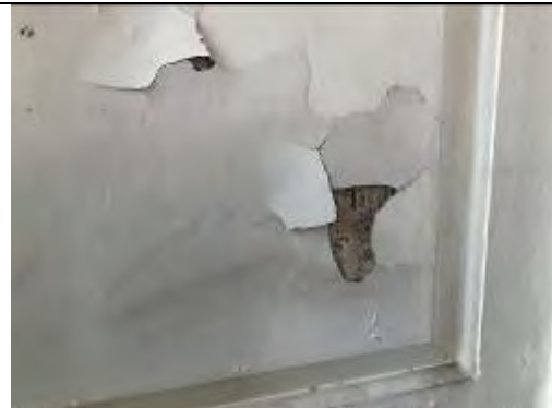
Plaster to be repaired
