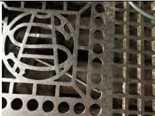
Cast pipes below floor grid
