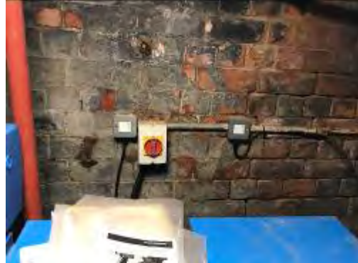
Debris to walls ASC/5 NADIS
