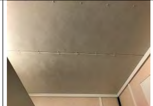
Modern non ACM boards to ceiling
