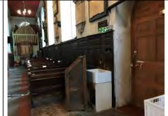
Slipped panels to be re fixed
