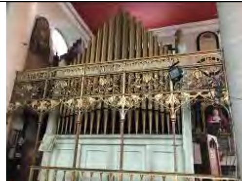
Presumed asbestos insulation board to blower box Crocidolite
