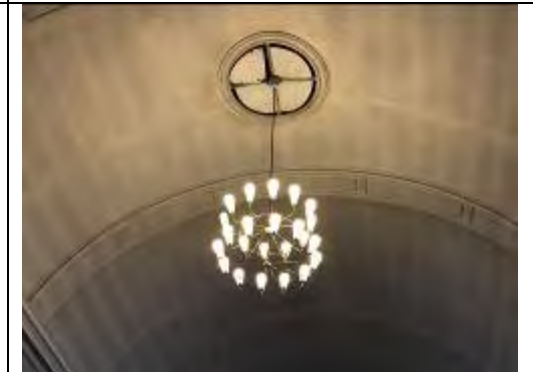
No Access to check boards to light fitting due to height
