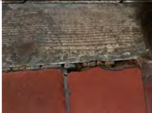
Timber to be removed
