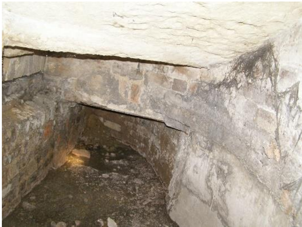
Fig 10 Duct going down to boiler room
