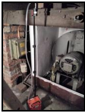
SP1 in operation with encapsulated panels in background
