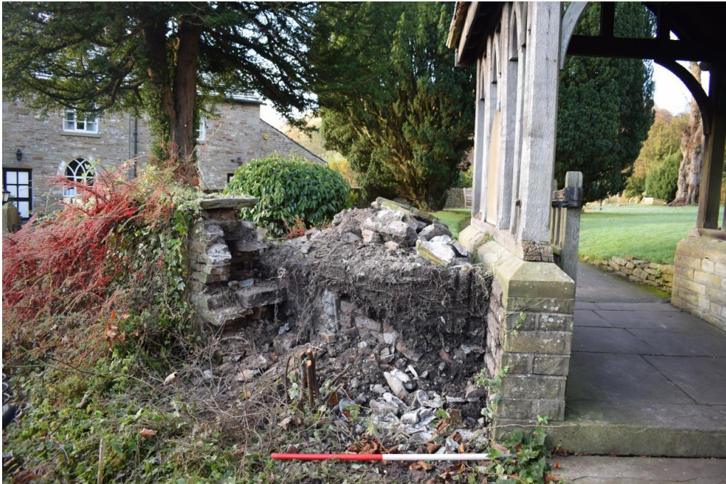
Figure 5 Wall removed at site of easy access ramp installation. Viewed from east. CPAT photo 4962-0001
