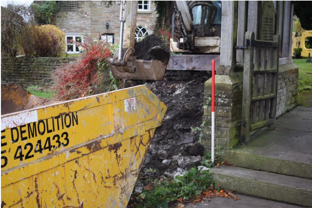
Figure 8 Excavation undertaken by 0.6 tonne mechanical excavator. Viewed from north east. CPAT photo 4962-0012
