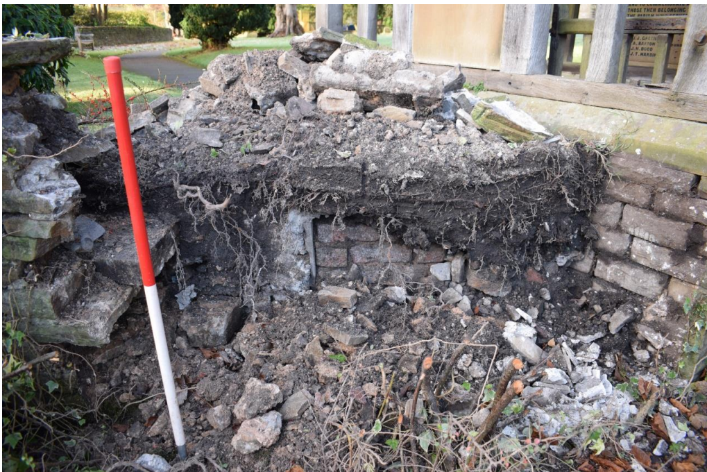
Figure 6 Wall removed at site of easy access ramp installation, detailed view of redeposited soil in situ. Viewed from south east. CPAT photo 4962-0005
