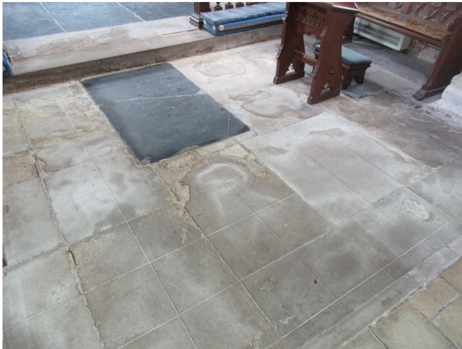
Fig.2, condition of the York stone floor, with a trip hazard against the ledger stone, normally covered by a carpet
