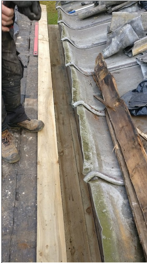
Photo 9. Repair to valley gutter between north aisle (right) and Willoughby Chapel, looking E.
