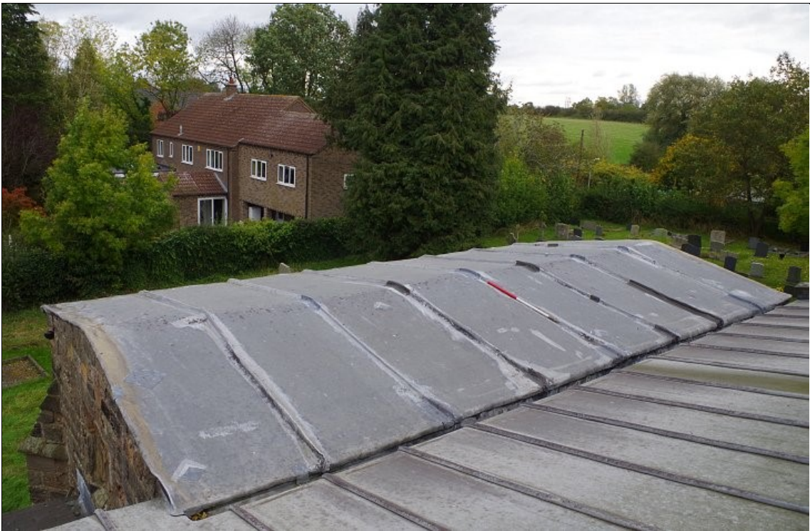
Photo 4. View of the lead roof of the Willoughby Chapel prior to replacement, looking NE.
