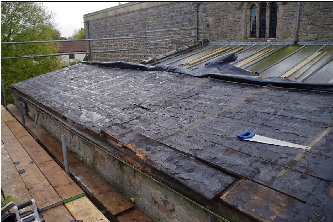
Photo 6. North slope of the Willoughby Chapel roof following removal of the lead, looking SE.
