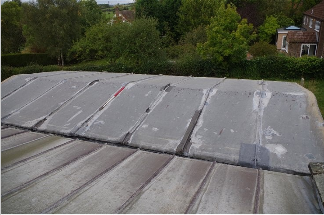
Photo 5. View of the lead roof of the Willoughby Chapel prior to replacement, looking NW.
