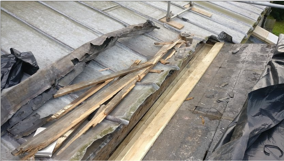
Photo 8. Repair to valley gutter between north aisle (left) and Willoughby Chapel, looking W.
