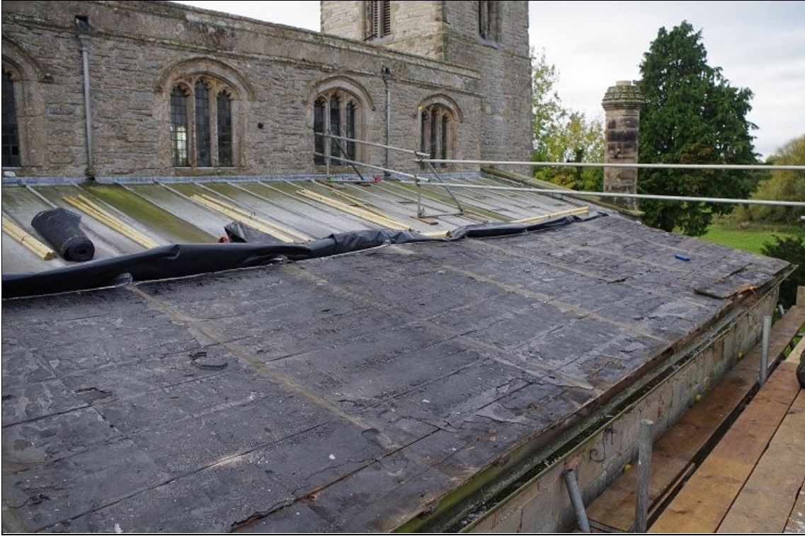
Photo 7. North slope of the Willoughby Chapel roof following removal of the lead, looking SW
