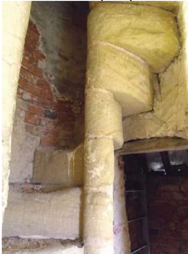
Figure 16 Remnant of spiral stairs within the main tower Note the top of the metal ladder on the right which is seen in Fig. 15 Picture credit: P R Associates, Design and Access Statement 2019
