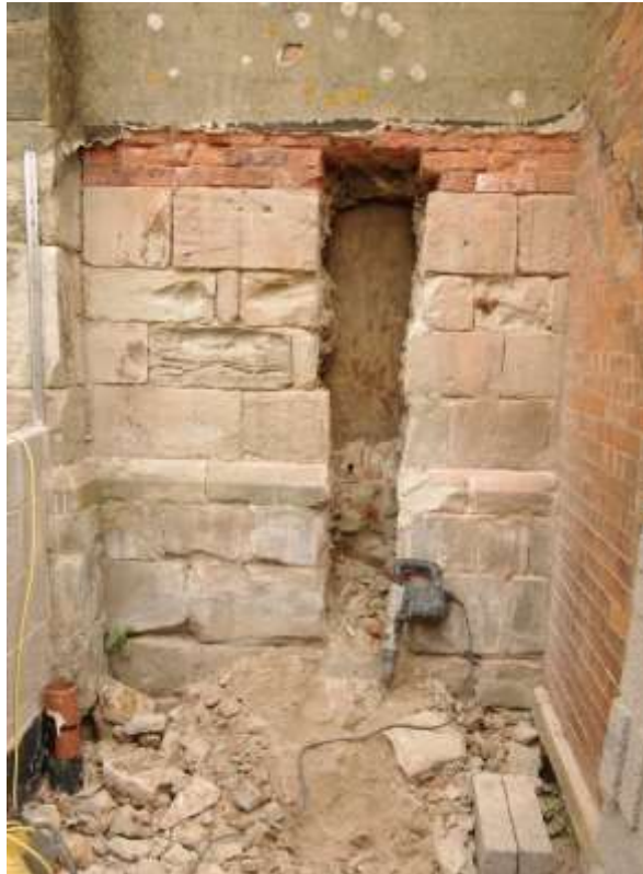
Figure 46 Full-height slot through tower wall The hole does penetrate through the wall although a board is against the inner face in this picture
