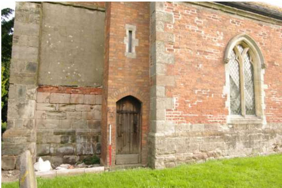
Figure 12 Location of proposed extension Looking north-east. 1m scale. Note the marks left by the demolished lean-to shed which had a roofline following the three courses of brick between the render and the stonework on the tower wall. The lean-to extended out as far as the brick-built clock and belfry access tower
