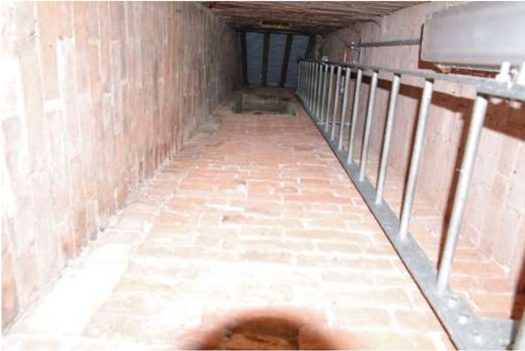
Figure 15 View up to the clock chamber and belfry access tower Looking north. The brickwork in the centre of the picture is part of the tower buttress. Note the infill of brick and later added wall on left. This indicates that the original tower access was within the main body of the tower – see Nichols illustration Fig. 3 and Fig. 16 below. This later access is probably from the 1867 remodelling
