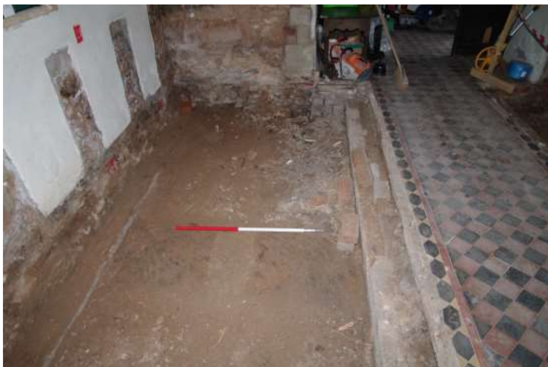
Figure 40 Compact layer beneath platforms Looking west on south side of aisle. The supporting bricks have been reduced in height down to the compact layer. 1m scale
