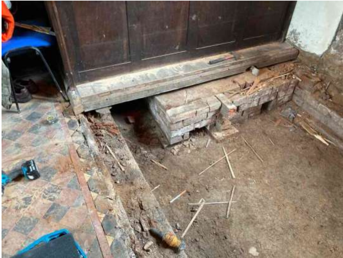
Figure 37 Exposed base for stove against south wall seen beneath pews Most of this plinth was left in-situ. Picture taken by Ackroyds
