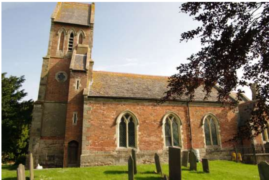
Figure 10 South facing elevation Looking south. 1m scale. The extension will be built against the base of the tower and wrap around the corner to finish at the left hand window (see Fig. 5)
