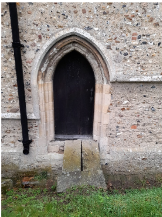
Water can pool in the brick lined gully.
