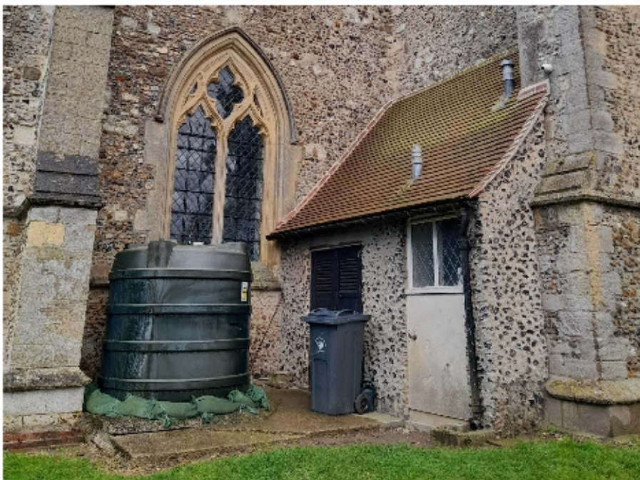
The current boiler room (behind black doors) may be too small to support a GSHP installation. The existing toilet is located behind the window. This structure could be removed after construction of the north side extension – alternatively the whole area could be used for heating plant.
