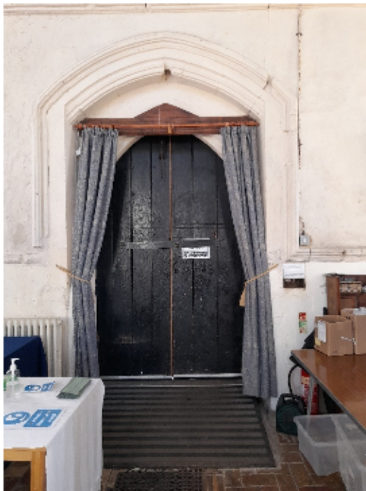
Main porch doors, proposed for provision of draught proof glass doors
