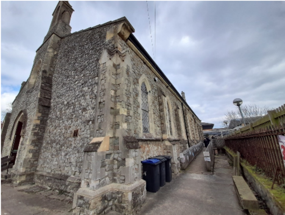
The south side of the building, ramp to the nursery with path to the boiler room next to the boundary fence. The roof is invisible from this angle.
