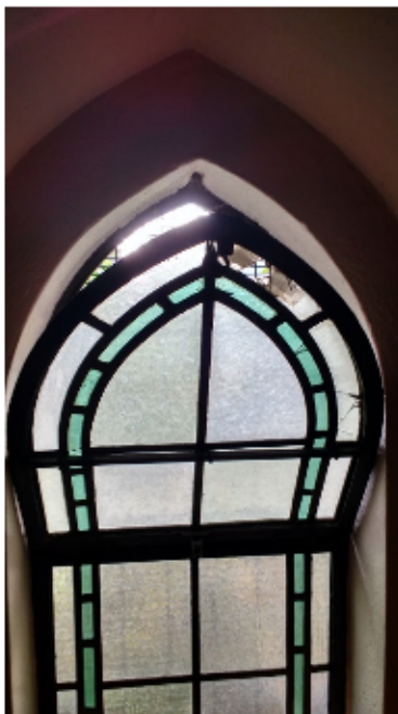
One of the vestry windows, above. broken.
