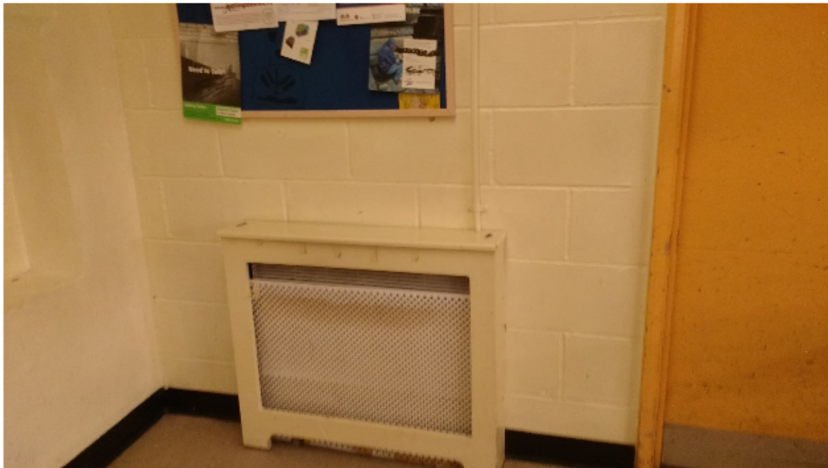
Electric heater in basement.
