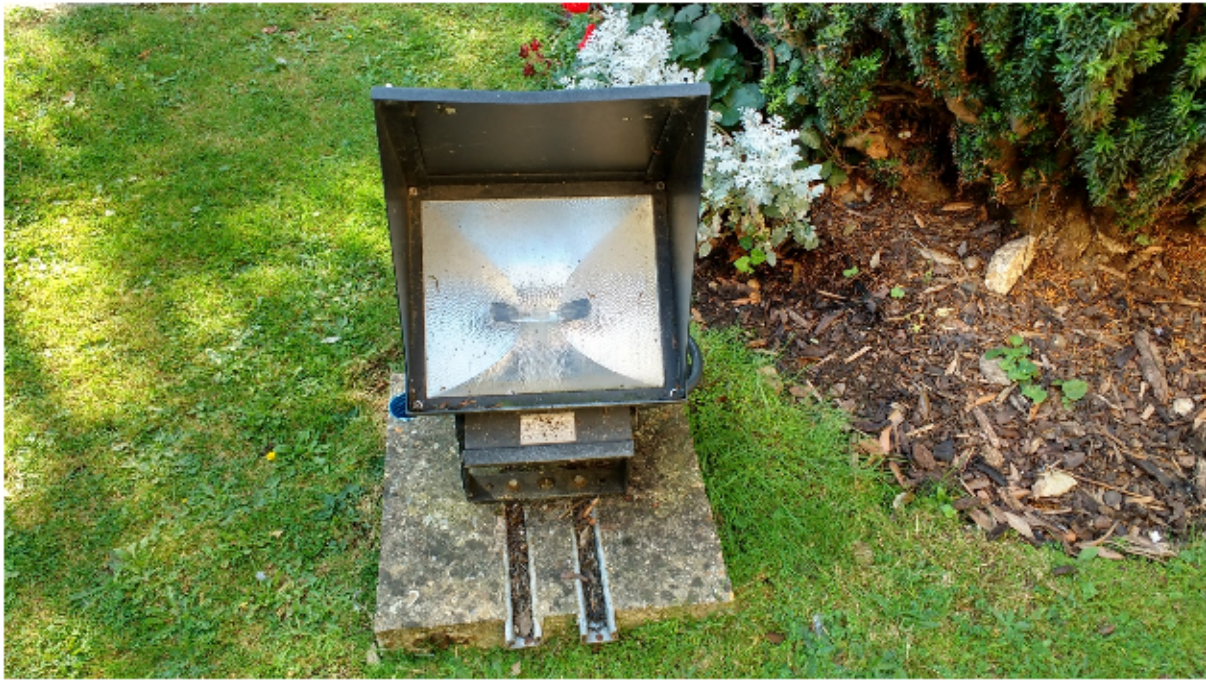
150W ground mounted floodlight – used occasionally
