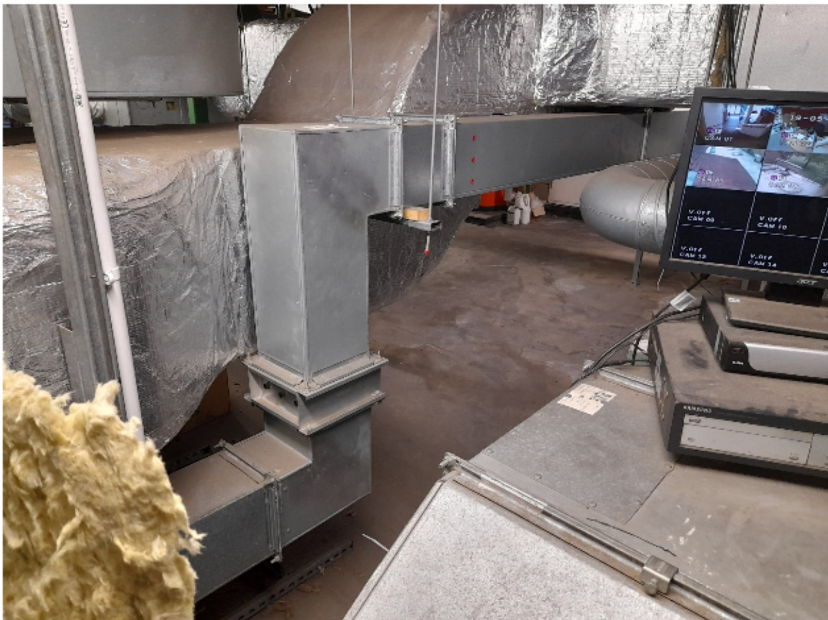
The boilers are located in the opposite corner of the room – the Hot Water boiler is the orange item in the centre of the image. Access involves squeezing into the gap between the ductwork
