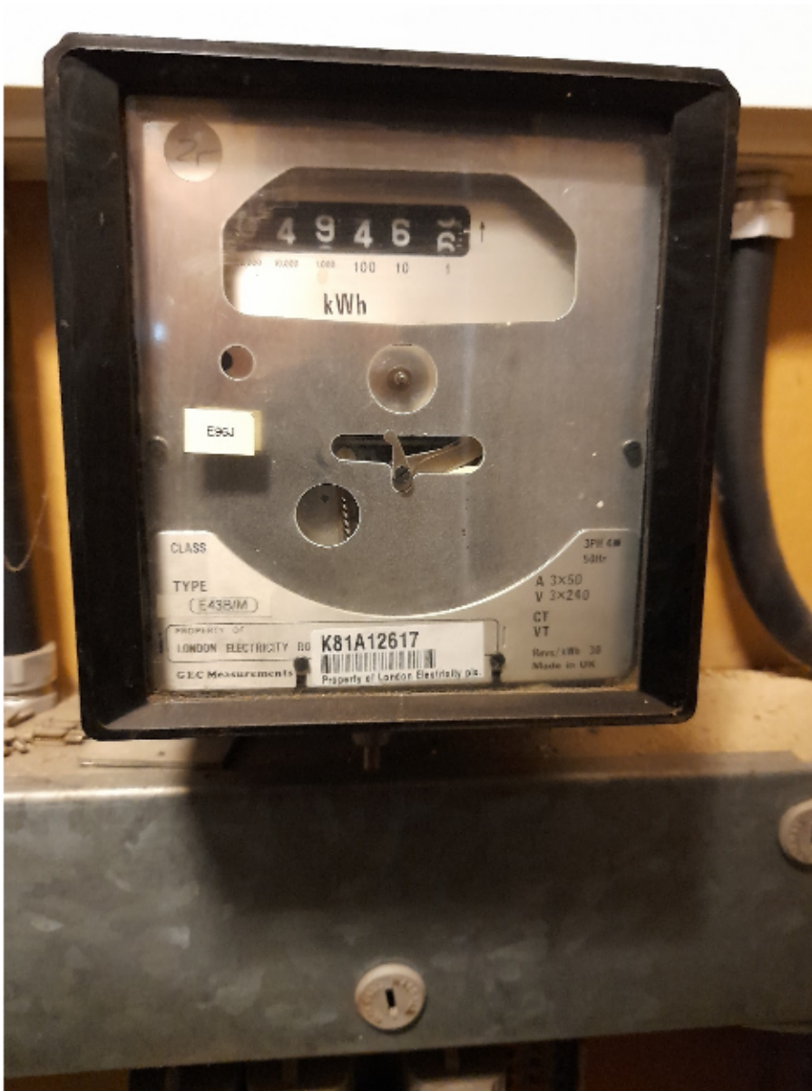
An electric submeter (which is not billed) is located in a plant room accessed from the crypt kitchen. Three phases of power are supplied.
