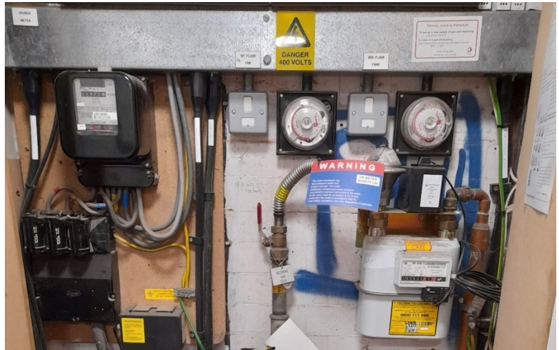
Three phases of power are provided.
