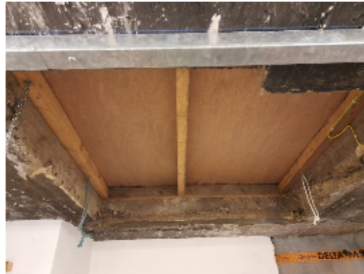
This feature above the basement store may be a trap door or an opening to a floor void
