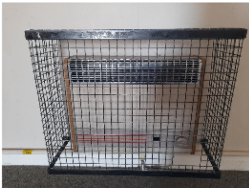
The existing gas heaters should be replaced.
