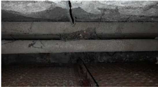
Under window voids with heating pipes.
