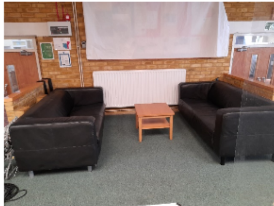
Area could benefit from instantaneous infra-red heating panels
