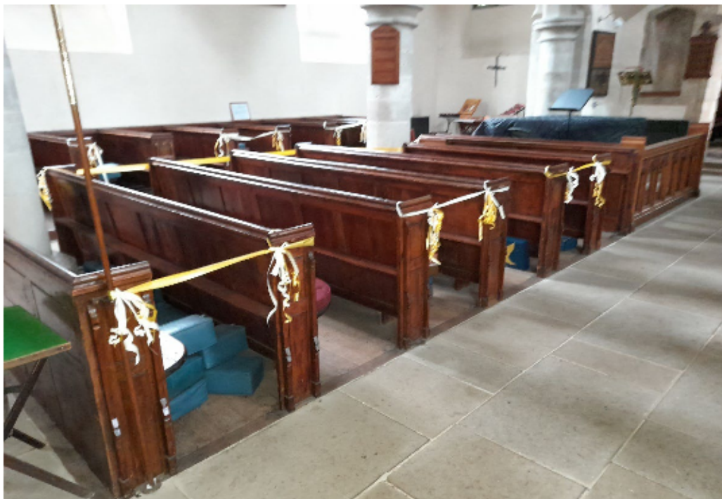
Under seat supports are fitted at various positions.
