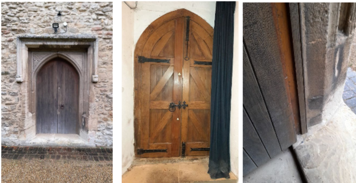
The tower door is wooden framed. It has no draught exclusion device underneath.
