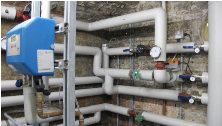
Figure 11 Boiler room pipework
