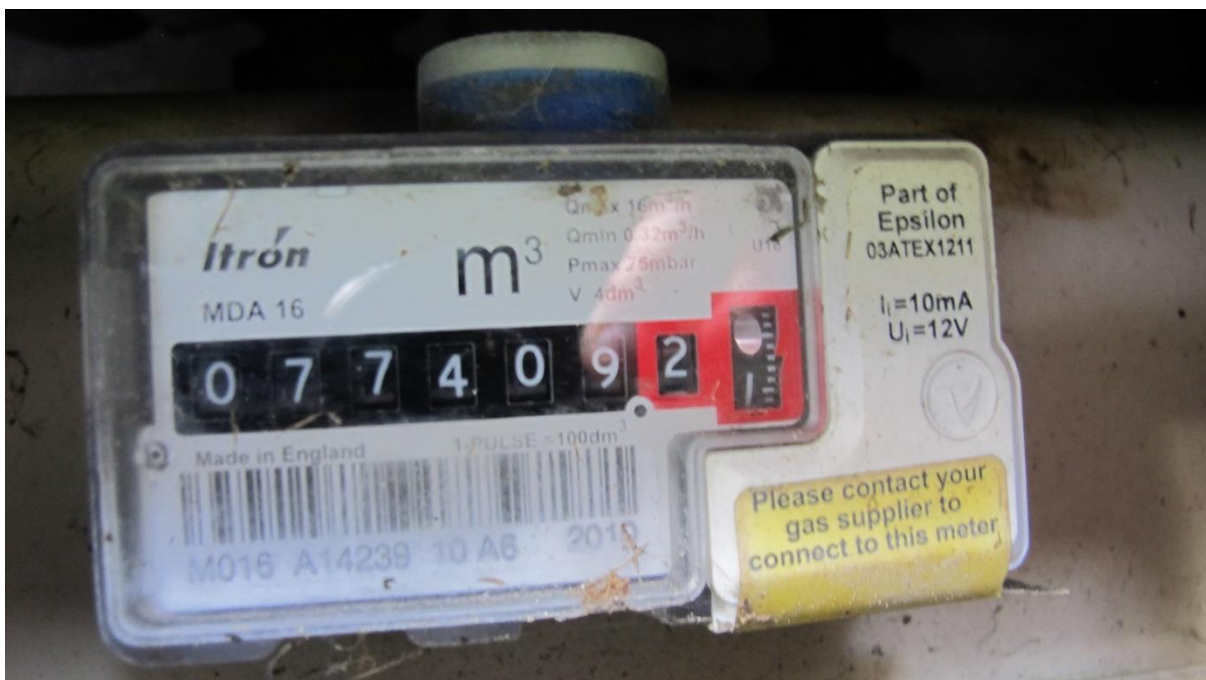
Figure 3. Gas meter is located in a cabinet against the NE building wall
