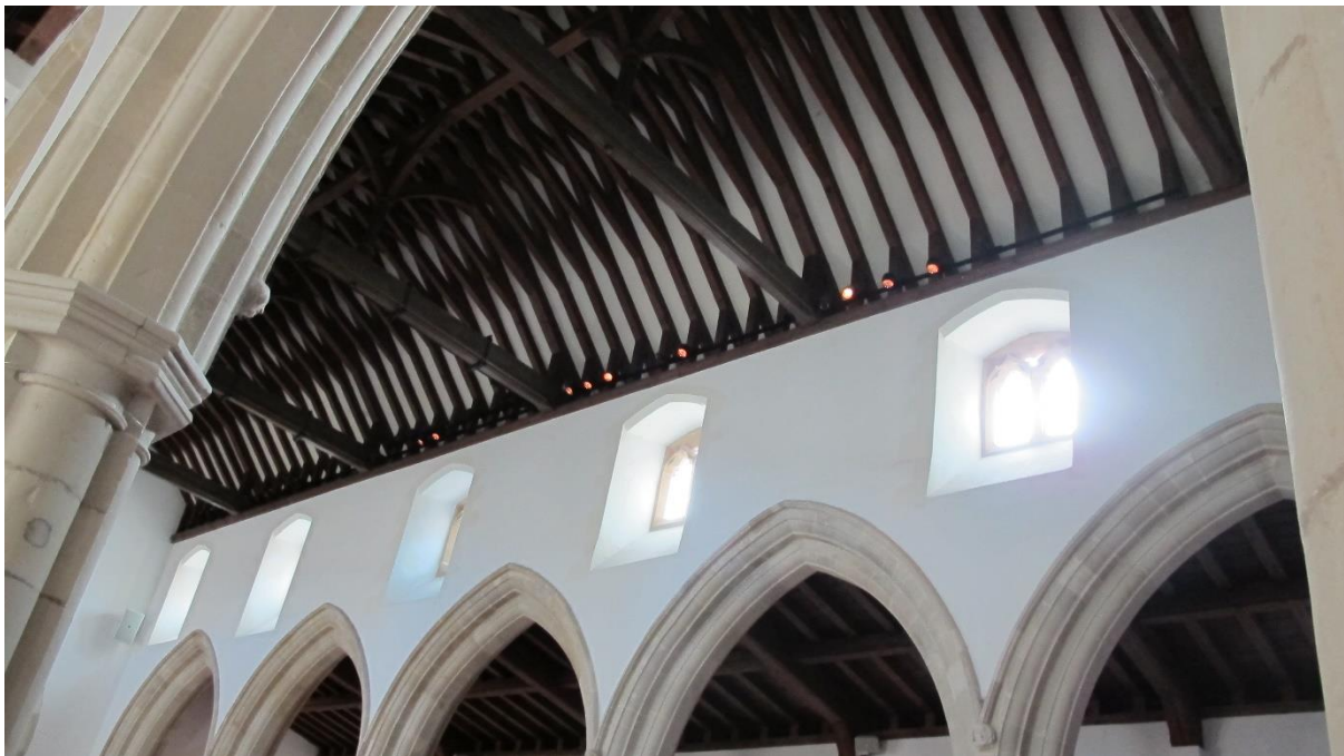
Figure 5 Location of nave lighting at base of roof
