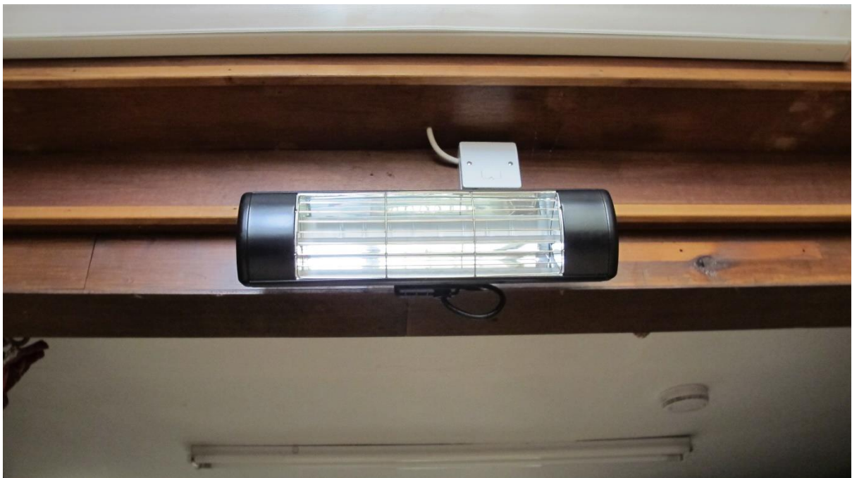
Figure 4 Vestry radiant heater
