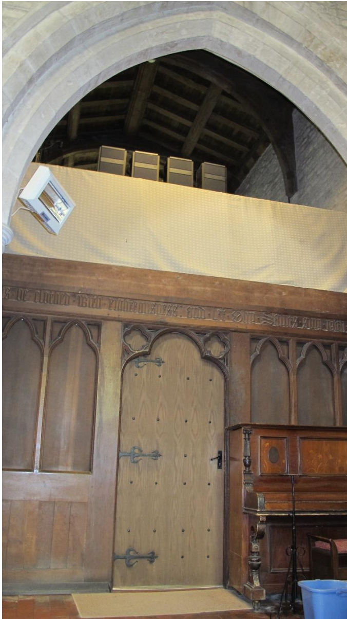
Figure 5 The vestry has a false ceiling. It was not possible to investigate the level of insulation above this. As the building is unheated for most of the time, insulation will not retain heat, so it may not be effective to add it. Is the radiant heater aimed at the pianist?
