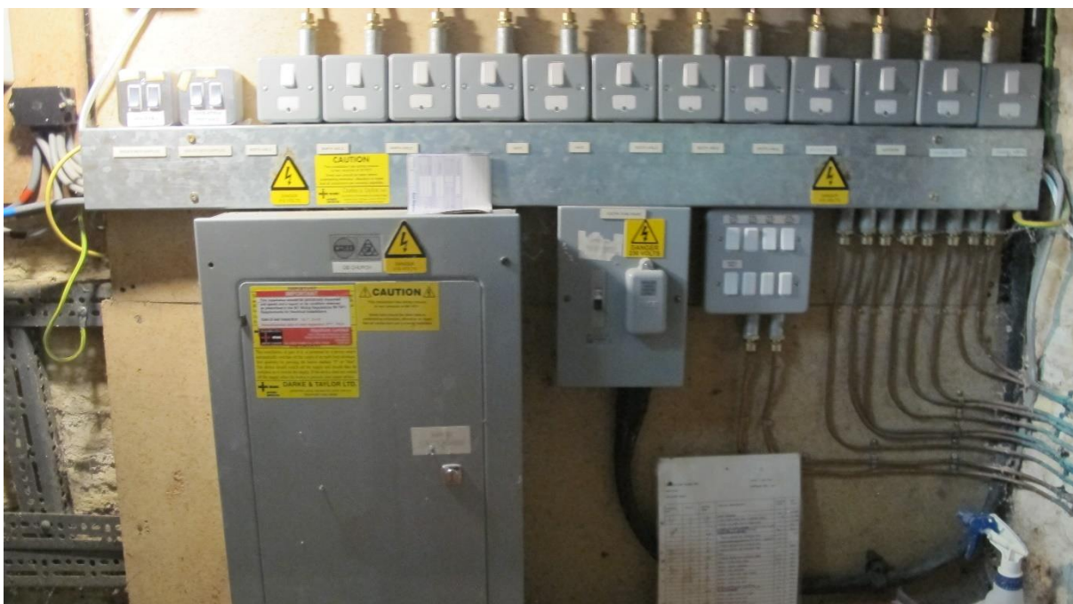
Figure 2 Independent switching of heaters (above) and lighting banks (lower right).
