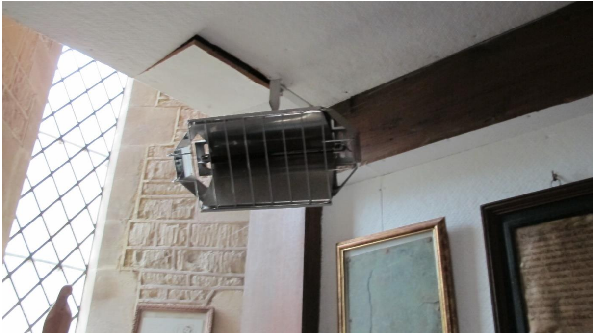
Figure 3 Vestry radiant heater
