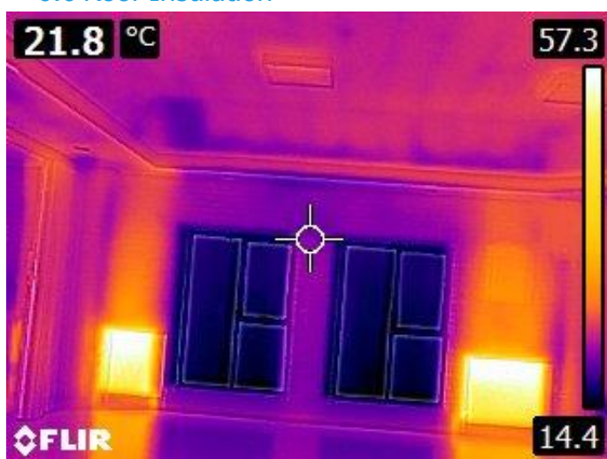
Photo 1 - Note darker areas near wall indicate missing insulation
